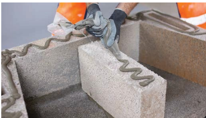
Press the middle section down on to the jointing adhesive and apply additional adhesive as shown.
