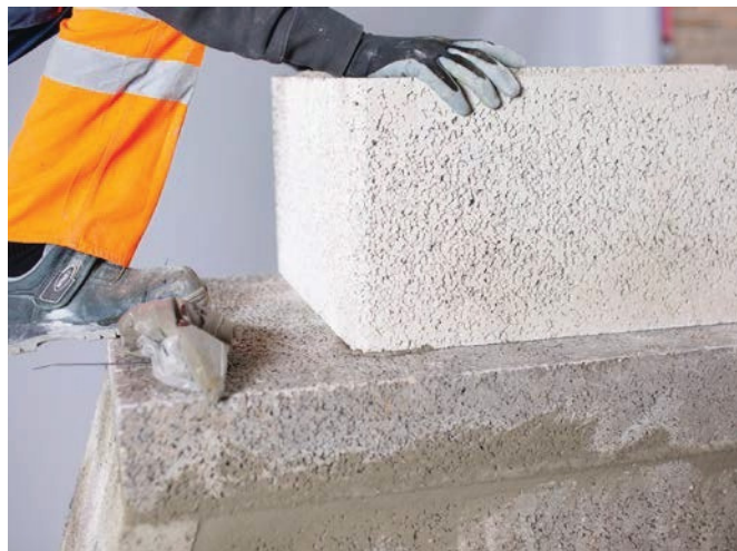
Press the first chimney block into place, checking it is in the correct position above the hole in the top plate.
